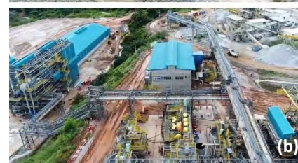
AMG's operations: (a) Mibra mine and (b) new spodumene plant (Photos: Courtesy of AMG)
